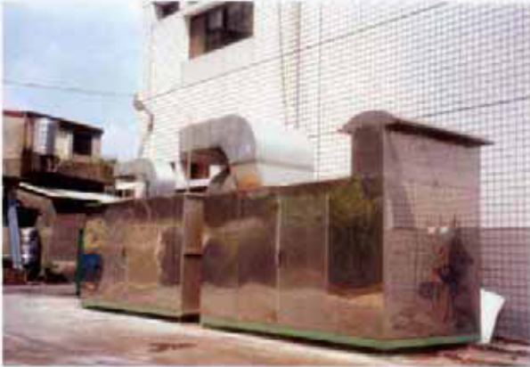
Air supplier and exhaust air system
